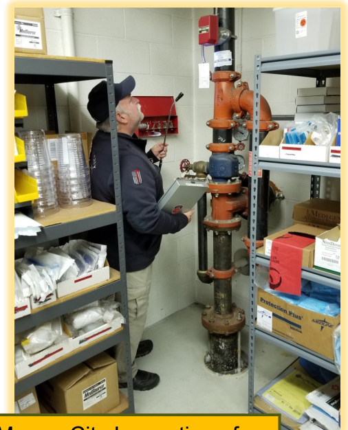
Murray City Inspection of a Fire Sprinkler Riser
